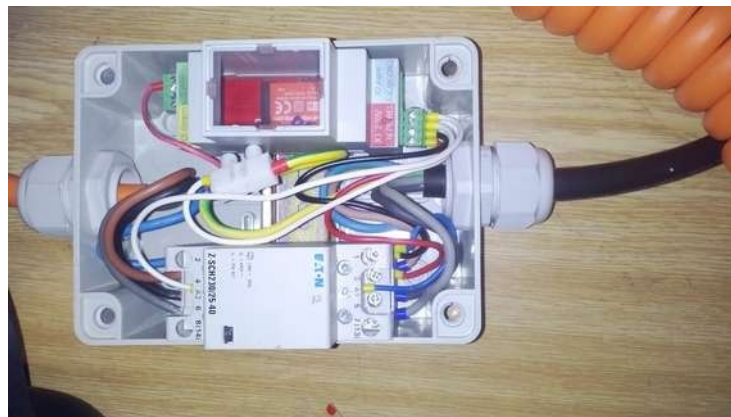
Picture 18: Charging cable made with EVSE DIN together with 4pole contactor in a box
